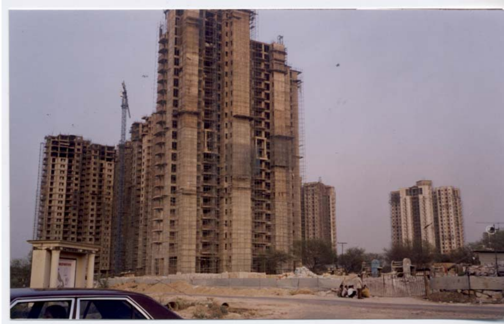
Hamilton Court & Regency Park using CLC block walls in DLF city near New Delhi (India)
