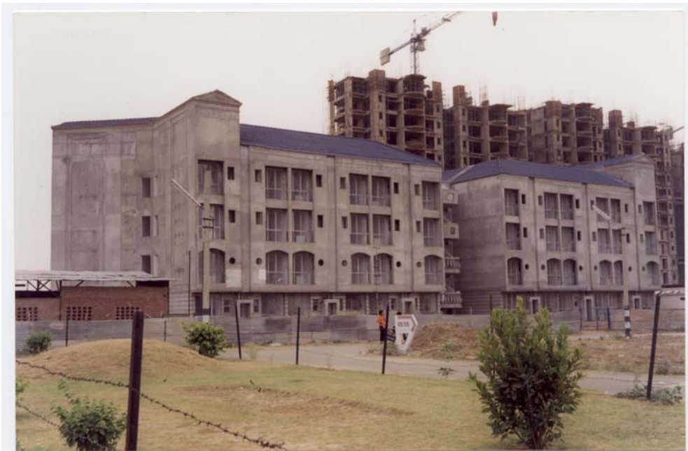
156 units of EWS dwellings with Cast in-situ Load-bearing Reinforced CLC walls of density 1200\text{kg/m}^3 - 1,600\text{ kg/m}^3 in DLF city near Delhi (India)
