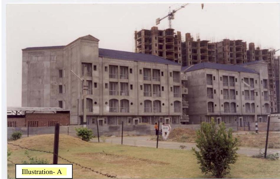
Reinforced CLC Load-bearing walls used for these 4-storey dwellings south of Delhi – 1997
